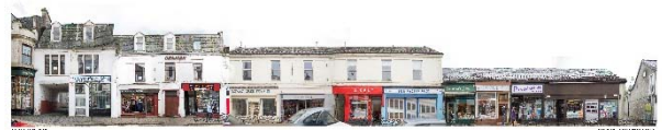
Streetscape photographs of Argyll Street showing condition of 2 and 3 storey buildings with varied roof profile and arrangements. Details include mansard roofs, dormer windows, parapet conditions, prominent gables, chimney stacks and brattishing.
